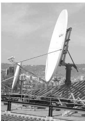
Fig. 4. View of the reception antenna installed in the ICC building
