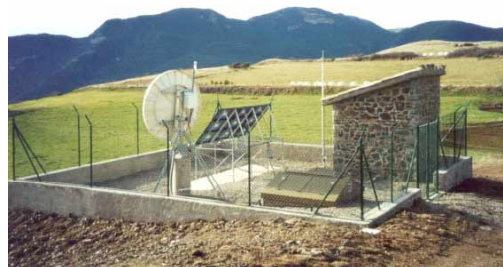
Figure 7. View of VSAT- Bruguera Station.
