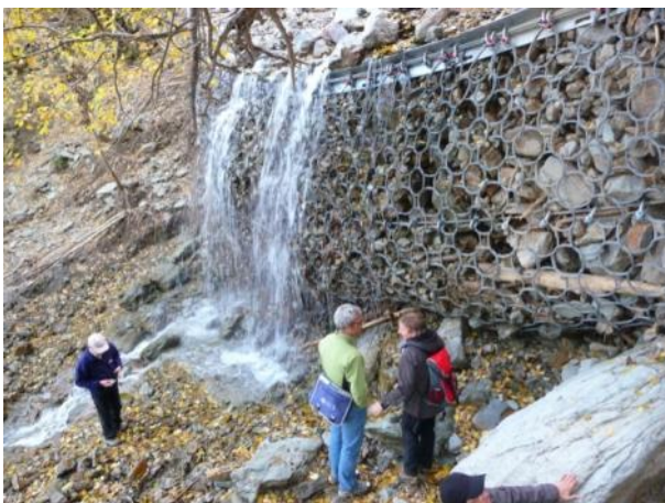
Figure 4 – Excursion site Portainé torrent with completely filled debris flow protection fences
